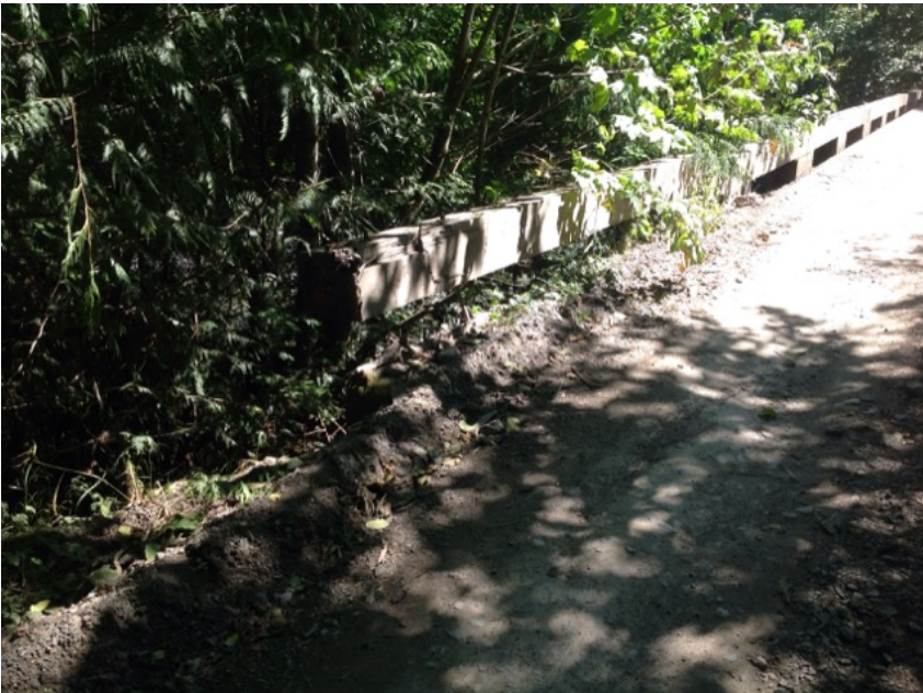
missing block on fender
