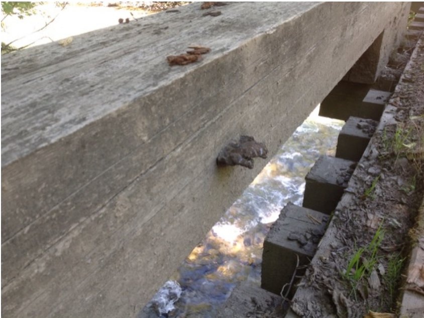
conk growing on guardrail
